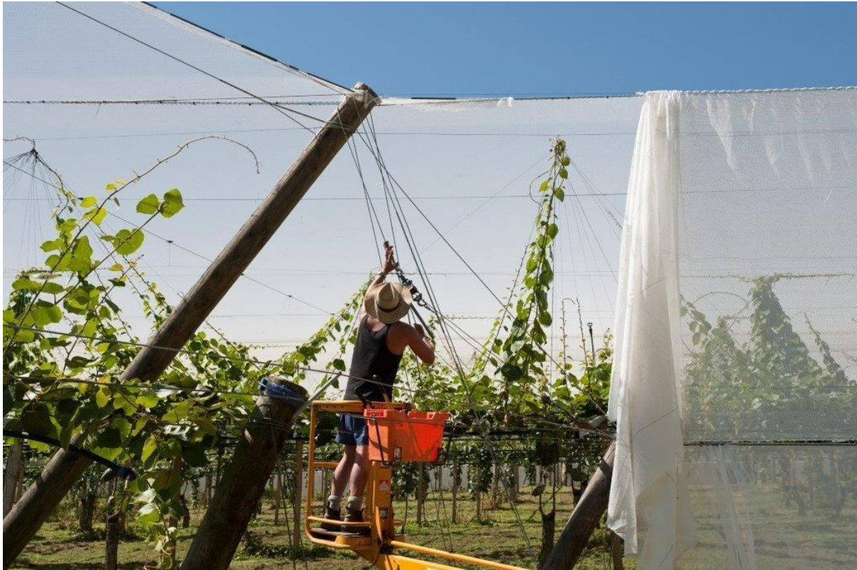
Image 15: The erection of hail netting over an orchard. In this instance the structure also has enclosed sides.
